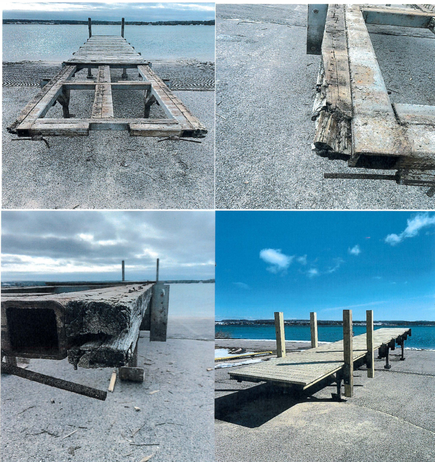
North Park dock pictures of wood in various stages of decay compared with new decking and posts being installed.
