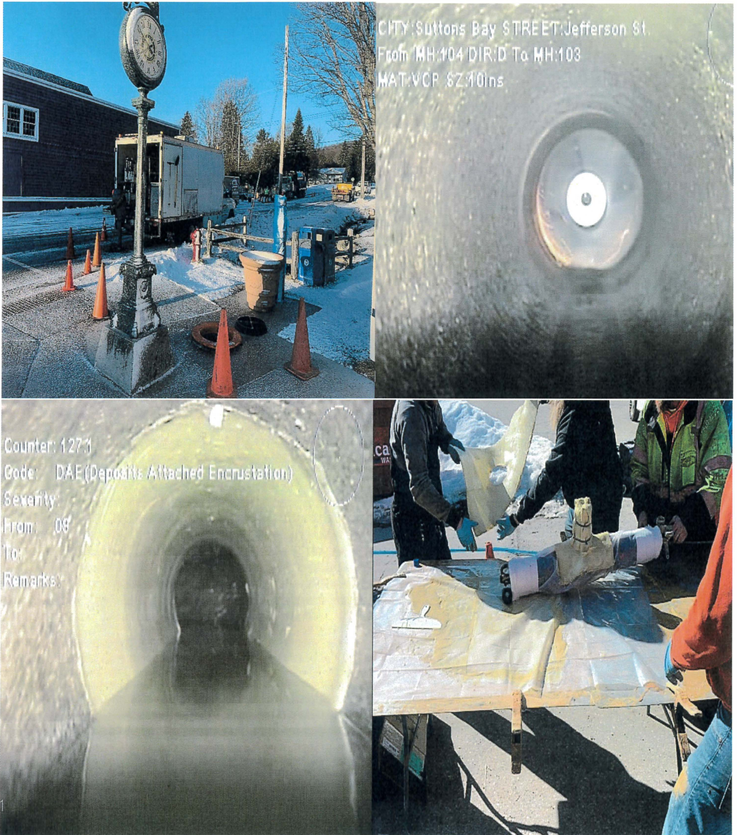
Top Row: Staging area on Jefferson St., sparks from grinding off calcium deposits due to leaks in pipe joints.
